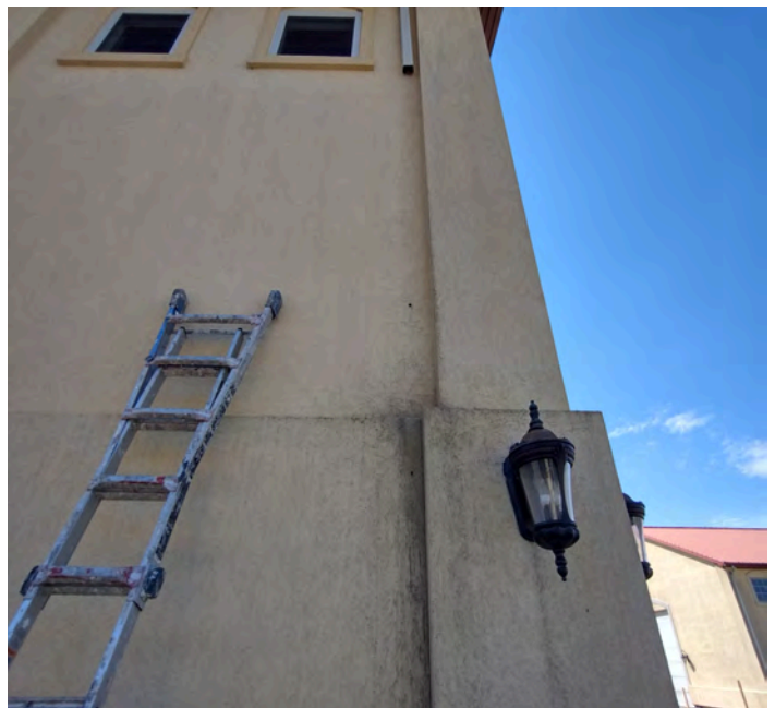
Impact damage and extensive lamina erosion
